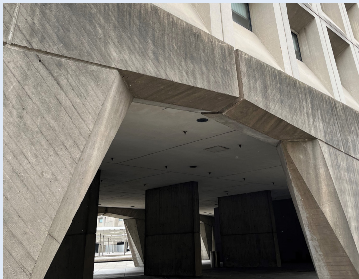
Figure 17: A building wall blackened over time by particulate matter in the air.
